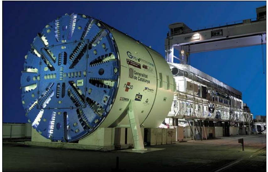
Illus. 2-This Tunnel Boring Machine, measuring approximately 39.5 feet (12.06 meters) high and showing its trailing support gear , was used in a project in Barcelona, Spain.
